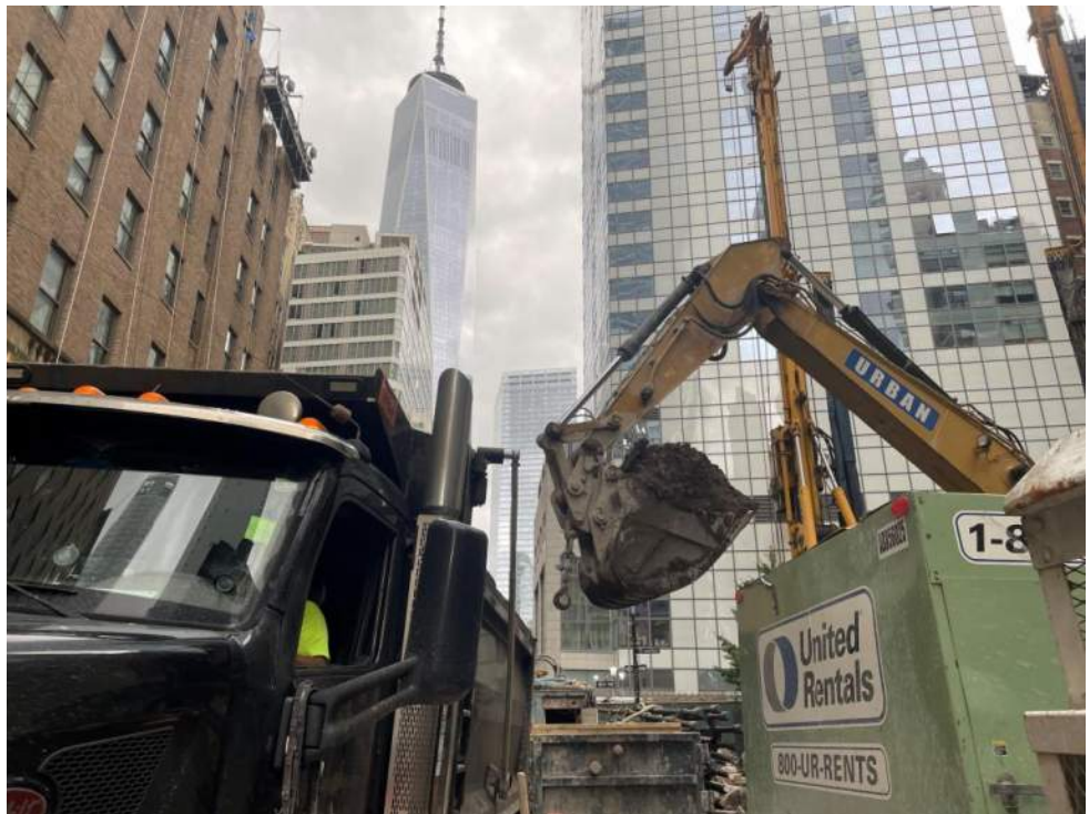
Photo 2: View of Urban loading truck with soil/fill for off-site disposal (facing north).
