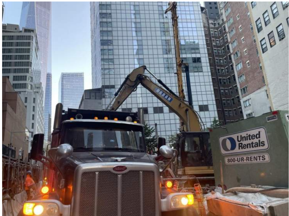
Photo 2: View of Urban loading a truck with soil/fill for off-site disposal (facing north).
