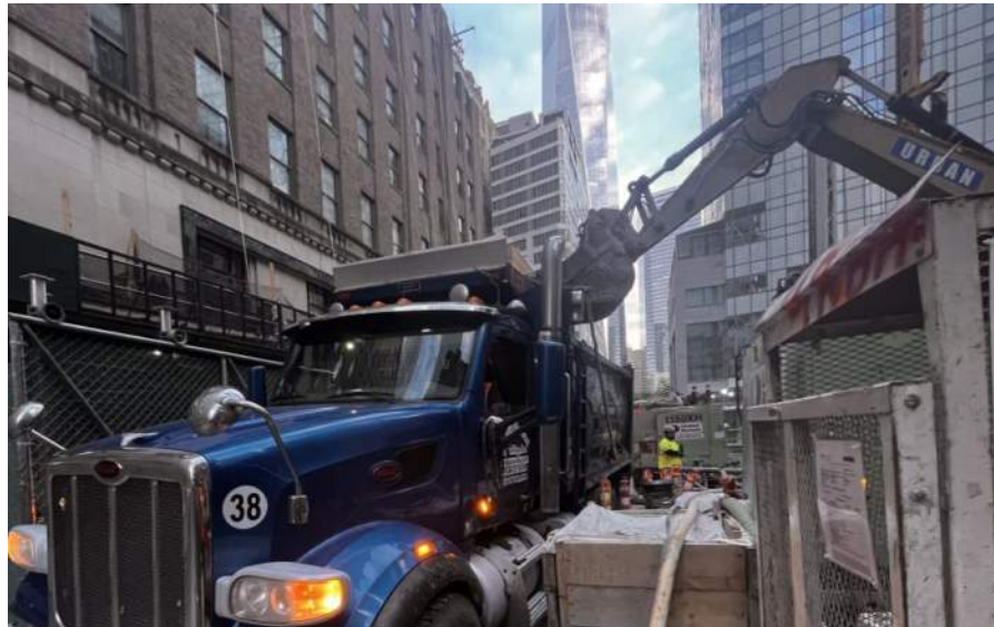
Photo 2: View of Urban loading a truck with excavated soil/fill for off-site disposal to the Bayshore Soil Management facility (facing north).
