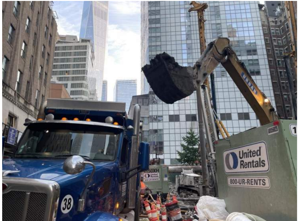
Photo 2: View of Urban loading a truck with excavated soil/fill for off-site disposal to the Bayshore Soil Management facility (facing north).
