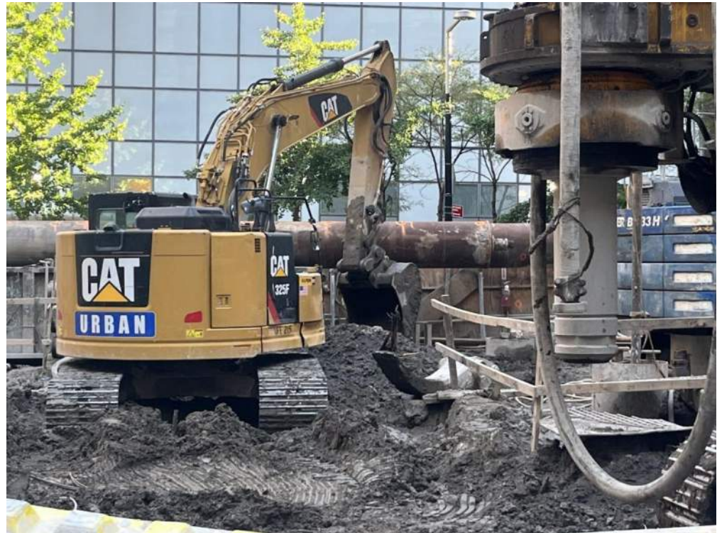
Photo 1: View of Urban excavating soil/fill in the northern part of the site (facing north).
