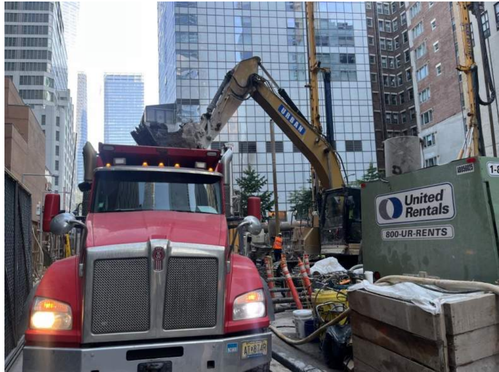
Photo 1: View of Urban loading a truck with soil/fill for off-site disposal (facing north).
