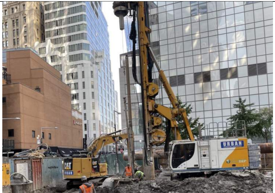
Photo 2: Urban advancing a caisson casing in the northern part of the site (facing north).
