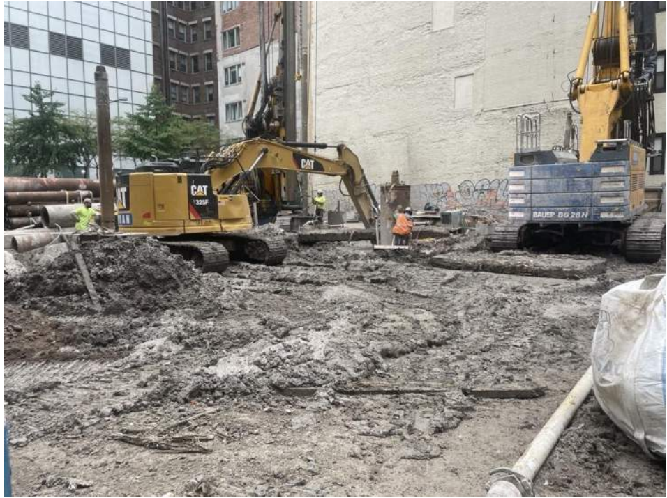
Photo 1: View of excavation of soil/fill in the southern part of WC03 (facing northeast).
