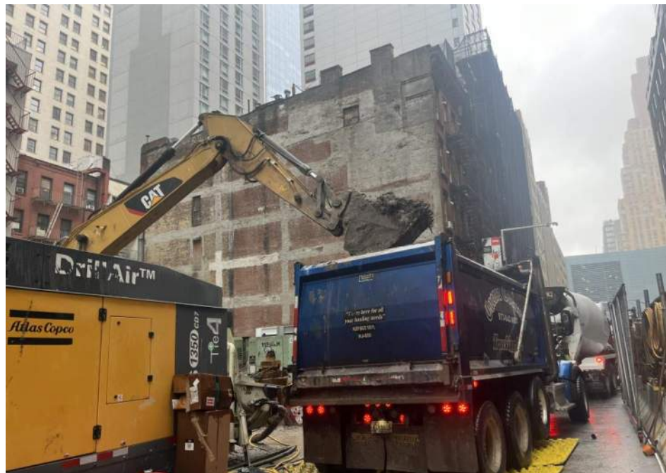
Photo 2: View of Urban loading a truck with soil/fill for off-site disposal (facing southeast).
