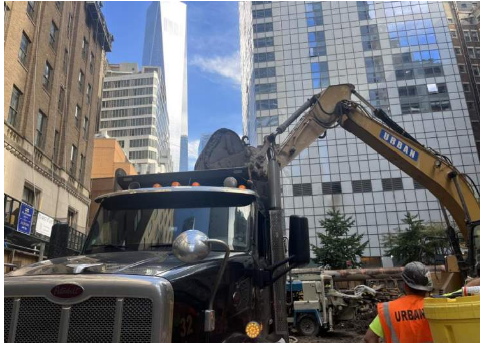
Photo 1: View of Urban loading a truck with soil/fill for off-site disposal to the Bayshore Soil Management facility (facing north).
