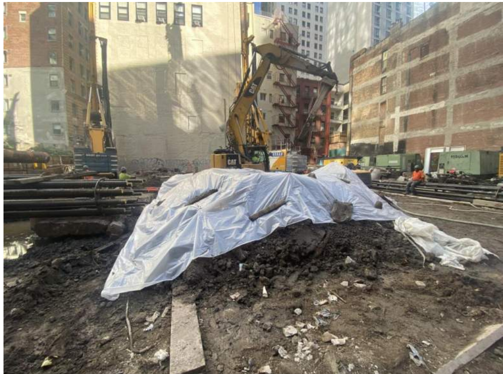
Photo 2: View of Urban covering the stockpiled soil/fill with polyethylene sheeting at the end of the day, pending off-site disposal (facing southeast).
