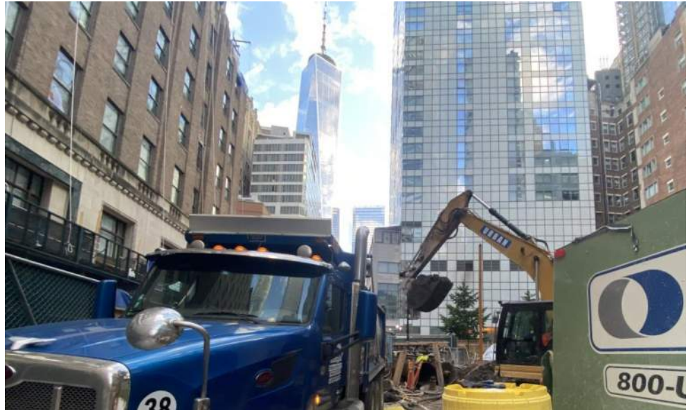
Photo 1: View of Urban loading a truck with soil/fill for off-site disposal to the Bayshore Soil Management facility (facing north).
