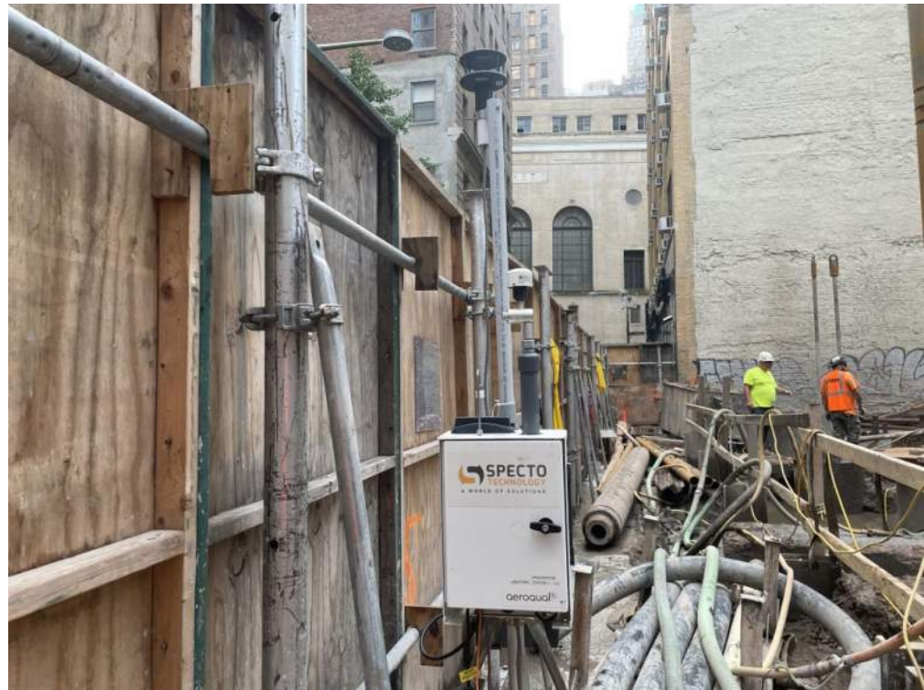
Photo 3: View of CAMP Station 1 in the northern part of the site (facing east).
