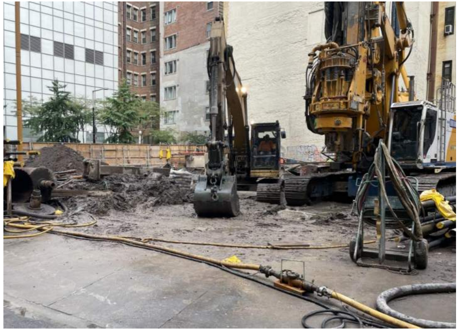
Photo 1: View of Urban grading soil/fill in waste characterization grid WC02 (facing northeast).
