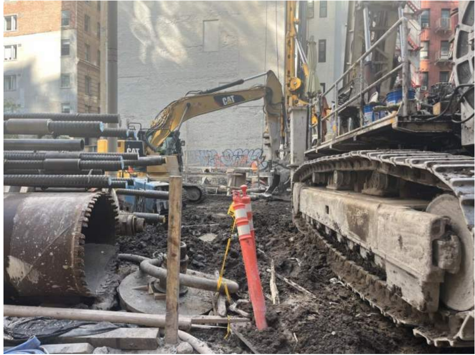
Photo 1: View of Urban grading soil/fill in waste characterization grid WC03 (facing east).
