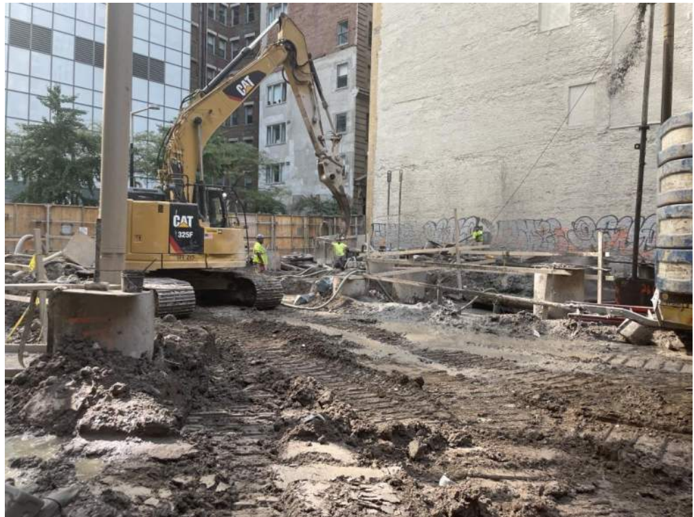
Photo 2: View of Urban excavating soil/fill in waste characterization grid WC03 (facing northeast).
