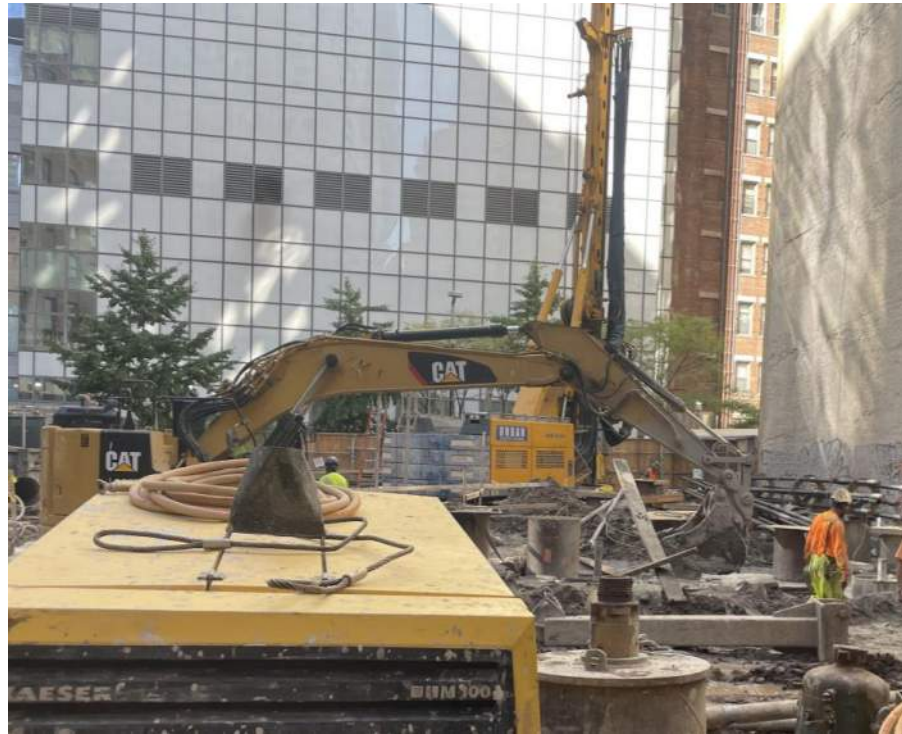
Photo 1: View of Urban grading in the southern part of the site (facing east).
