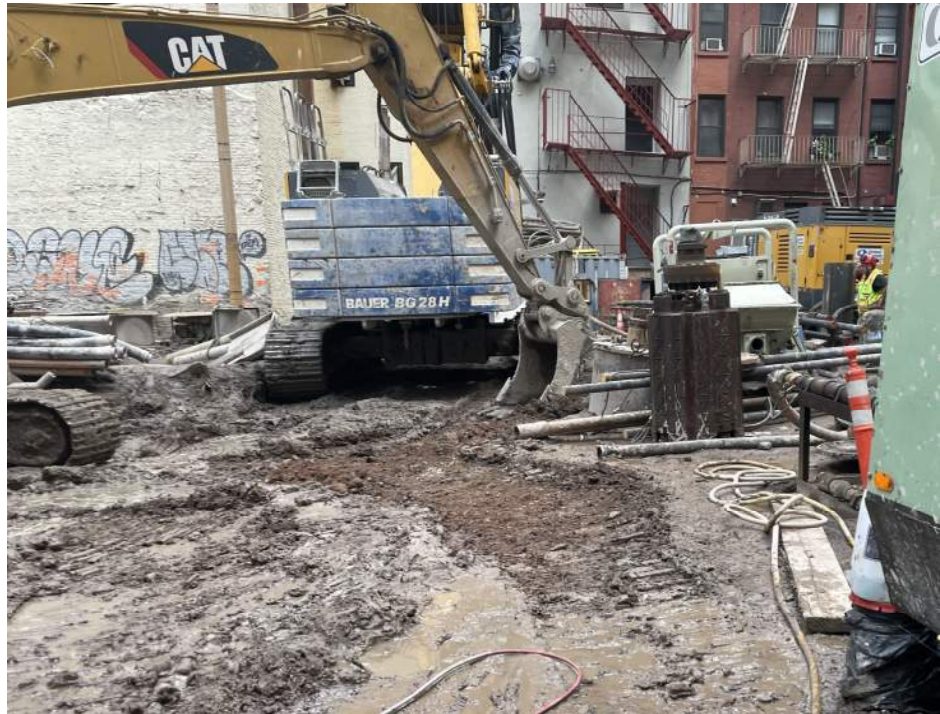
Photo 1: View of Urban grading in the southern part of the site (facing east).
