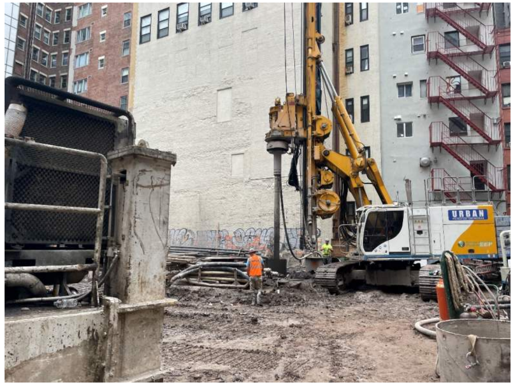
Photo 2: View of Urban drilling a rock socket in the eastern part of the site (facing east).
