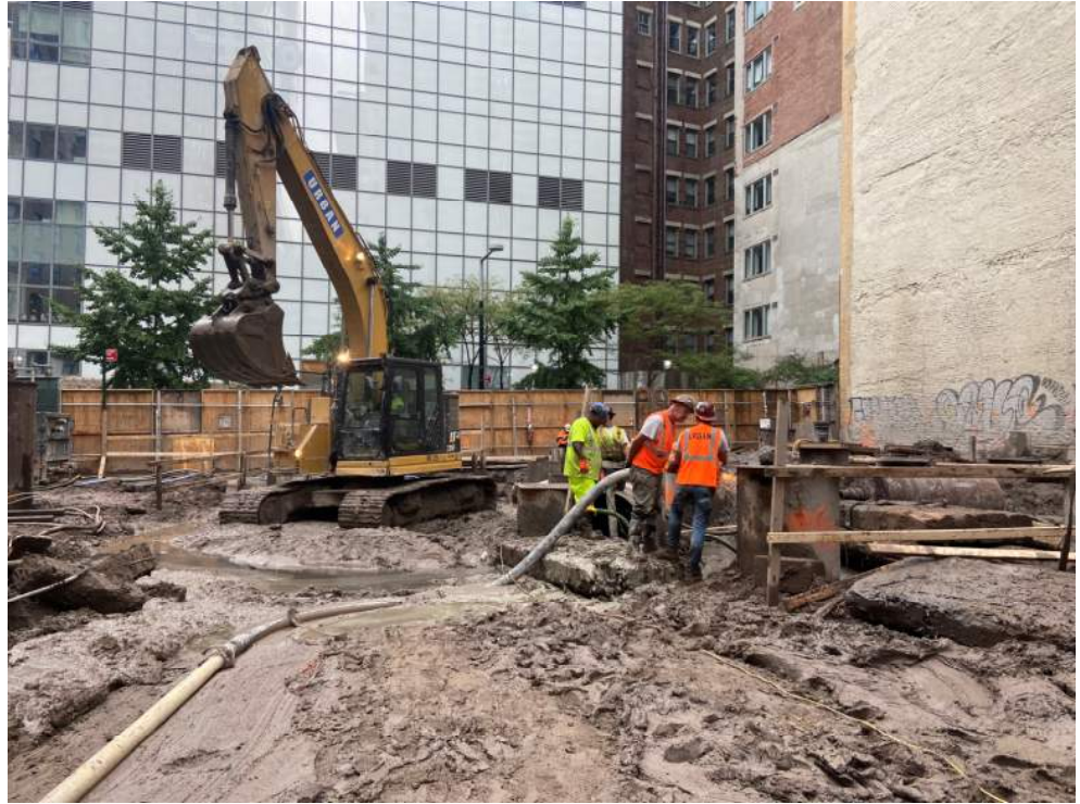
Photo 1: View of Urban grading soil/fill and placing grout in a caisson at the central portion of the site (facing north).
