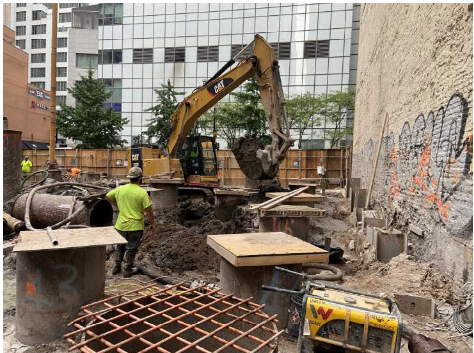
Photo 2: View of Urban excavating an about 10-foot-long by 10-foot-wide area to a depth of about 4 feet bgs in waste characterization grid WC03 (facing north).
