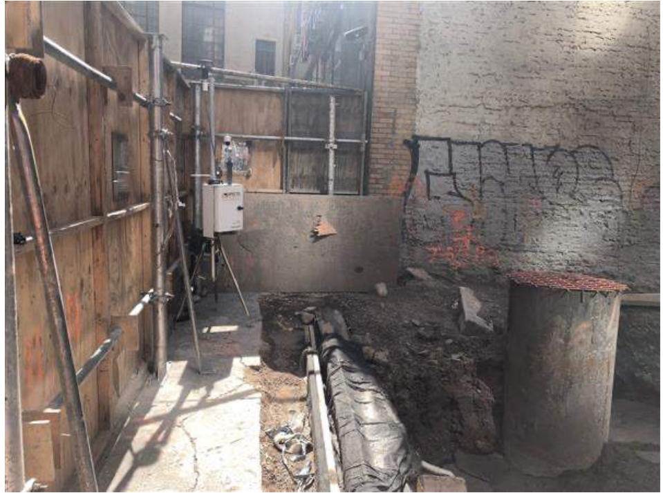
Photo 3: View of CAMP Station 1 in the northeastern part of the site (facing east).
