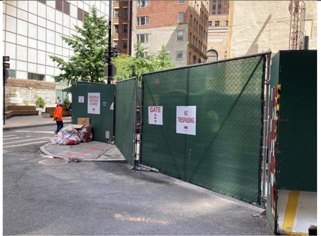
Photo 4: View of the entrance/exit of the site along Washington Street at the end of the work day (facing northeast).
