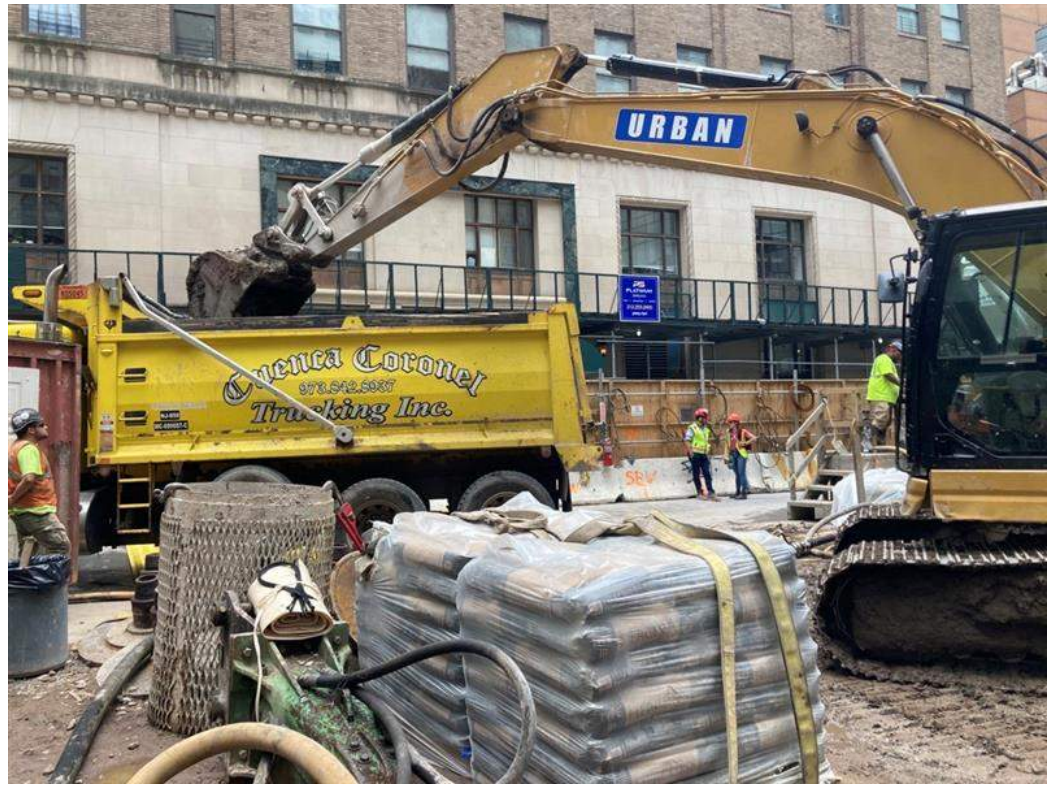
Photo 1: Urban loading a truck with non-hazardous soil/fill for off-site disposal (facing northwest).
