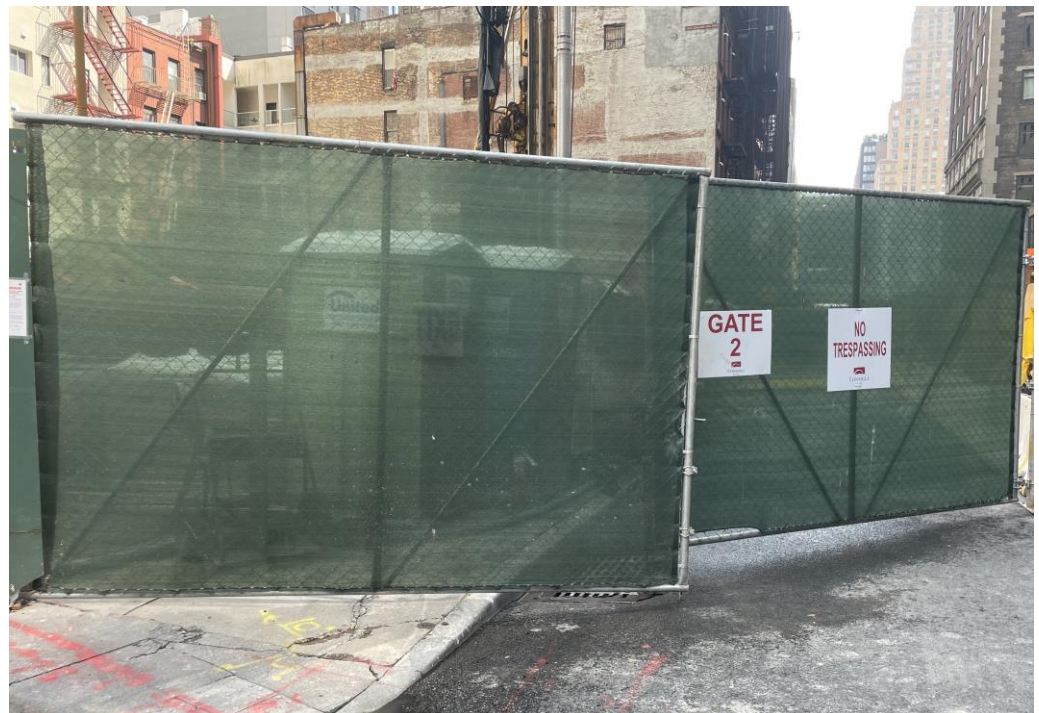
Photo 6: View of the entrance/exit of the site at the corner of Washington and Carlisle Street at the end of the work day (facing southeast).
