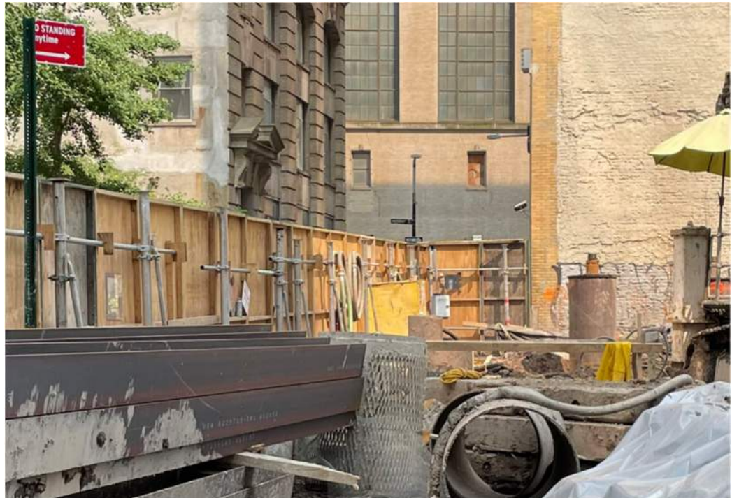
Photo 4: View of CAMP Station 1 (next to the construction fence) in the northeastern part of the site (facing east).
