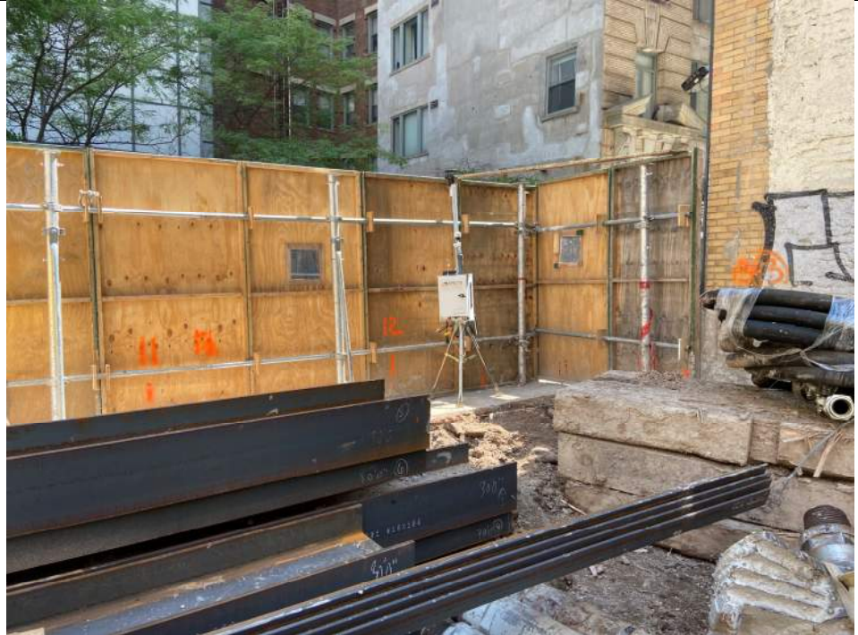
Photo 3: View of CAMP Station 1 in the northeastern part of the site (facing northeast).
