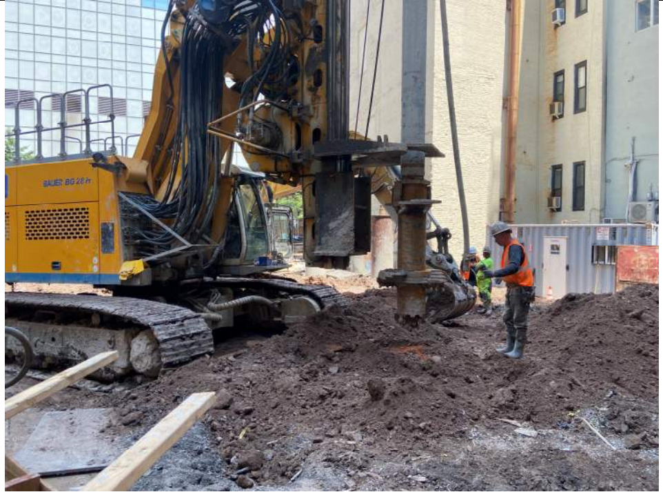
Photo 1: Urban preparing for the installation of a soil-mix column in the southern part of the site (facing northeast).
