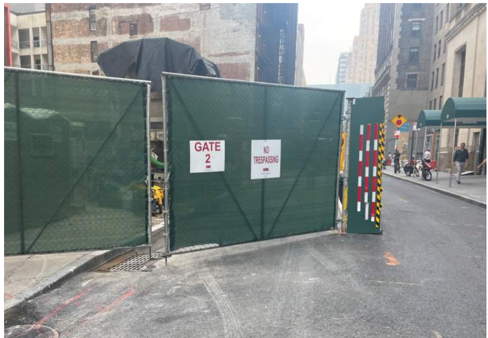
Photo 6: View of the entrance/exit of the site at the corner of Carlisle and Washington Street at the end of the work day (facing south).
