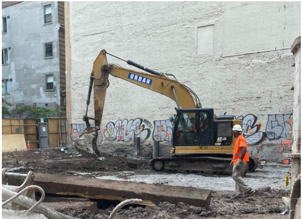
Photo 1: Urban grading soil/fill in the central part of waste characterization grid WC03 (facing northeast).
