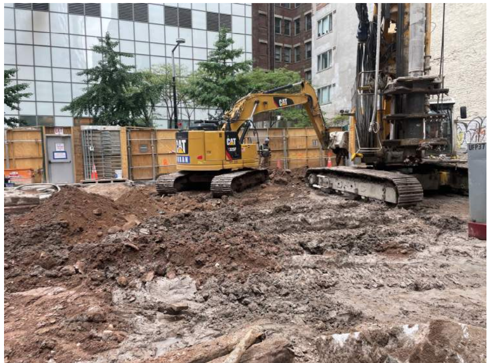
Photo 2: Urban excavating soil/fill in the northern part of waste characterization grid WC03 (facing northeast).
