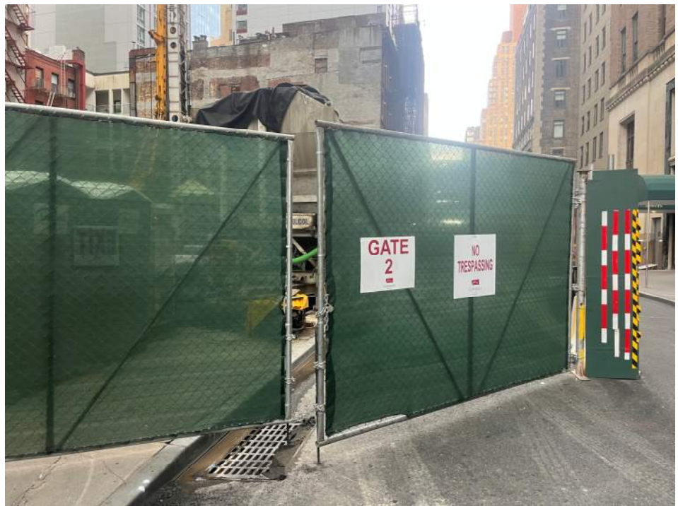
Photo 6: View of the entrance/exit of the site at the corner of Carlisle and Washington Street at the end of the work day (facing south).
