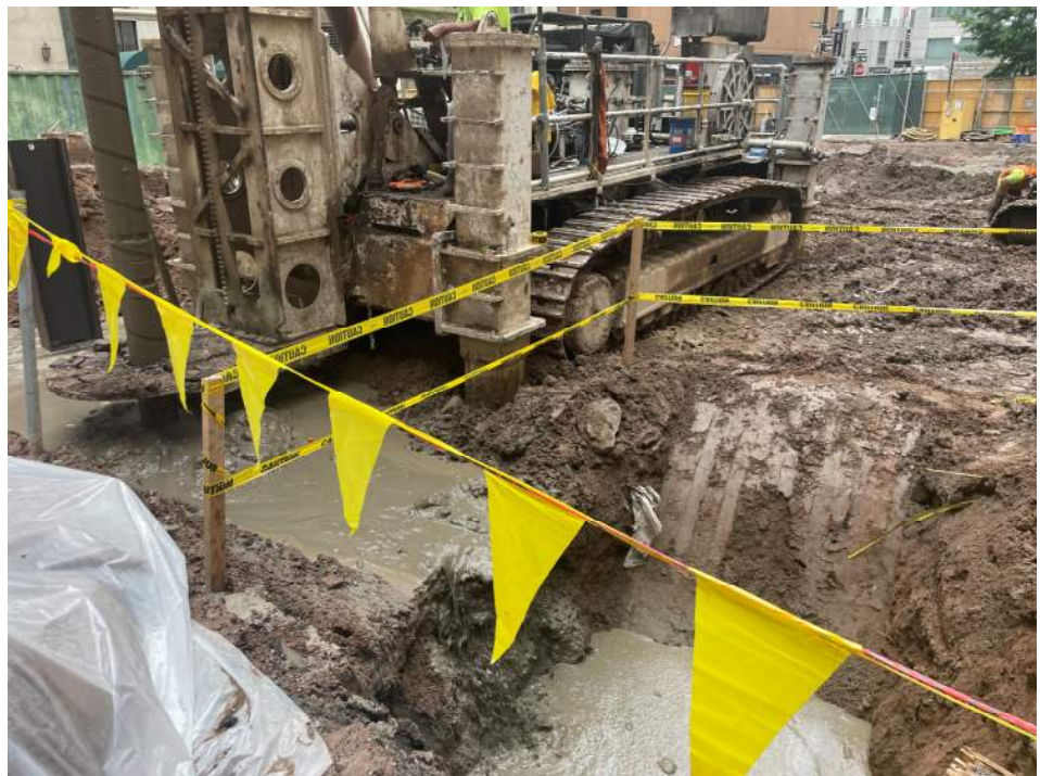
Photo 2: Urban installing soil-mix columns as part of the ISS in the southern part of the waste characterization grid WC04 (facing northwest).
