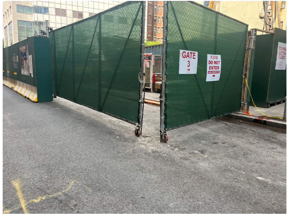
Photo 5: View of the entrance/exit of the site along Washington Street at the end of the work day (facing northeast).
