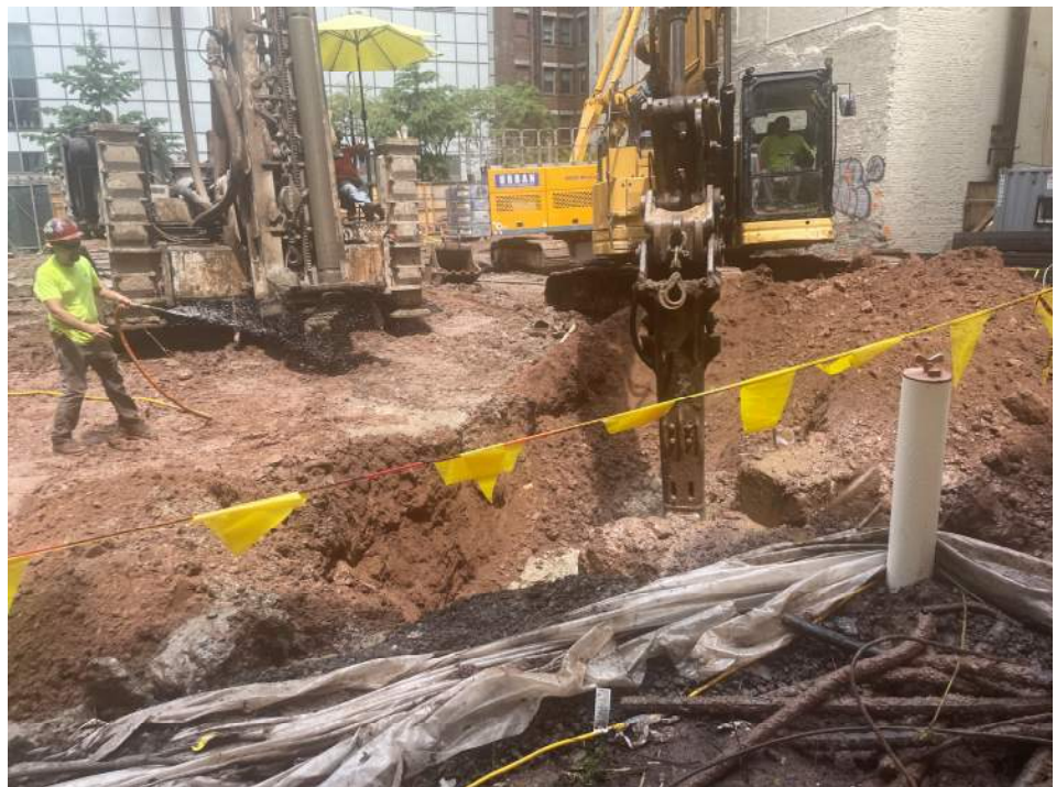
Photo 2: Urban using a hose for dust suppression while breaking up concrete in the southern part of the site (facing northeast).
