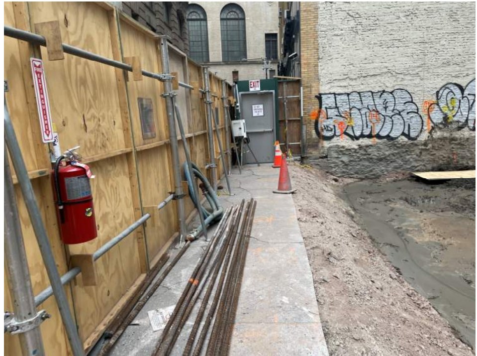
Photo 5: View of CAMP Station 1 in the northern part of the site (next to door) (facing east).
