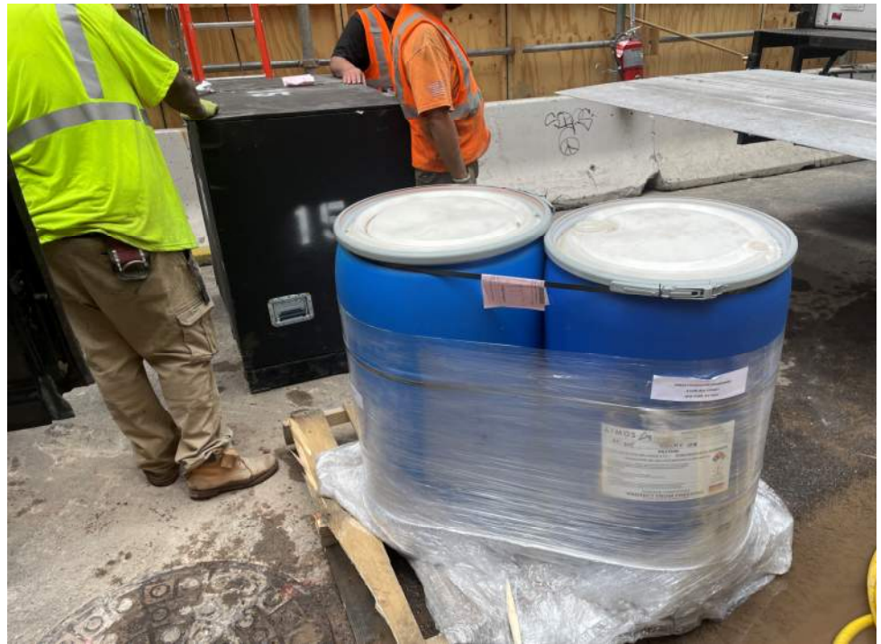
Photo 3: View odor suppressant foam delivered to the site for use during UST cleaning, decommissioning, and removal (facing west).
