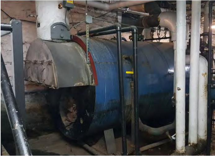
BOILER IN BASEMENT
