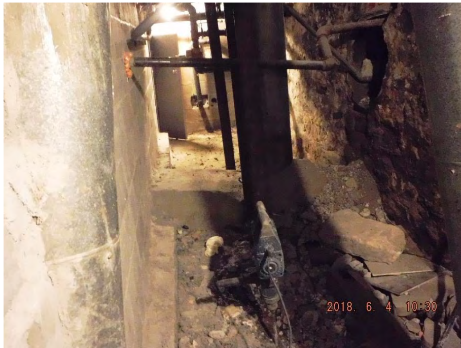
Photograph 2: Locations of B2 and B3. B3 was installed at far end of room. Tank vault at left. Dry cleaning machine support columns shown
