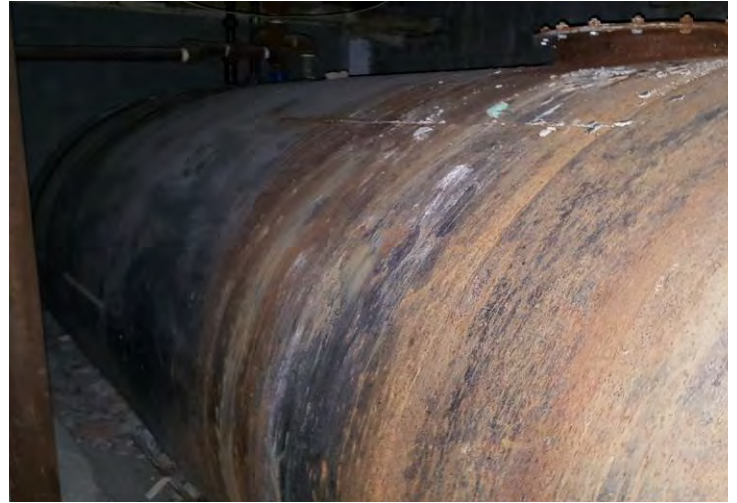
6,000-GALLON AST IN BASEMENT
