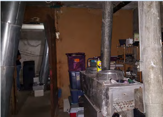
SUPPORTS IN BASEMENT INDICATIVE OF A DRY-CLEANER
