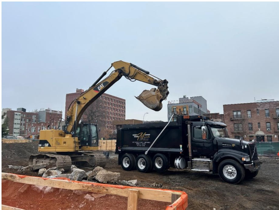
Photo 2: View of contractor loading C&D for off-site disposal in Lot 53, facing east.
