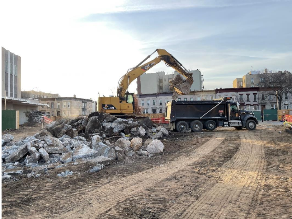
Photo 1: View of contractor loading C&D for off-site disposal on Lot 14, facing south.
