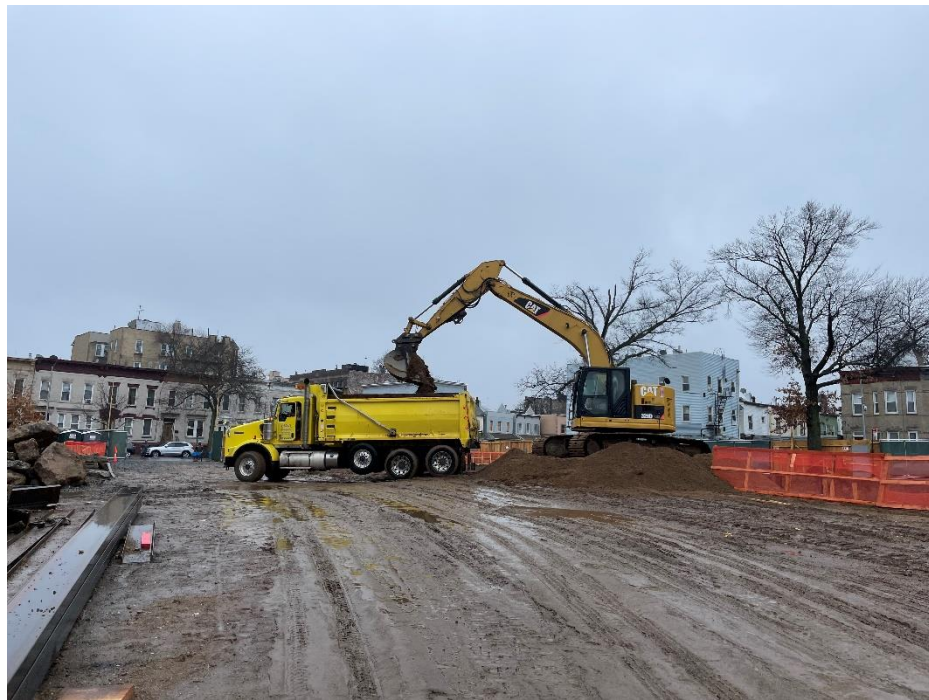
Photo 2: View of contractor loading soil for off-site disposal on Lot 14, facing south-southwest.
