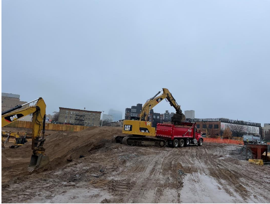
Photo 1: View of contractor loading soil for off-site disposal on Lot 14, facing northeast.
