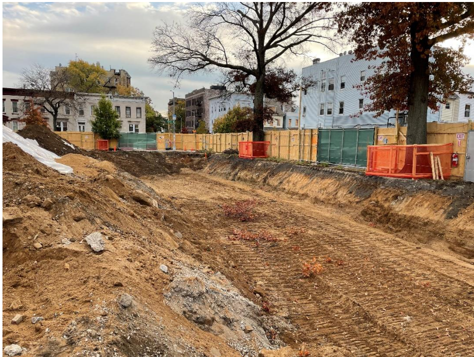
Photo 2: View of excavation for SOE installation along the perimeter of Lot 14, facing southwest.
