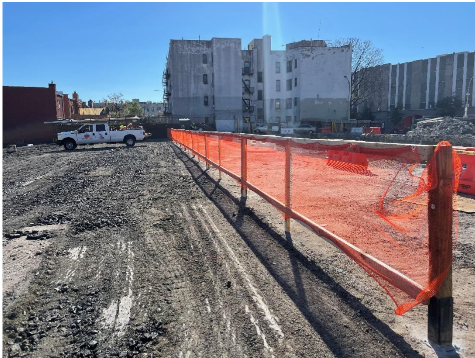
Photo 2: View of contractor installing SOE guardrail along the perimeter of Lot 53, facing south.
