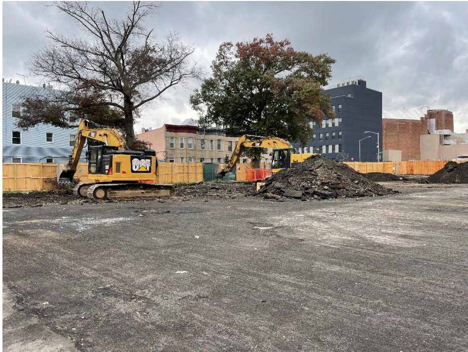
Photo 1: View of excavation for SOE installation along the perimeter of Lot 14, facing northwest.
