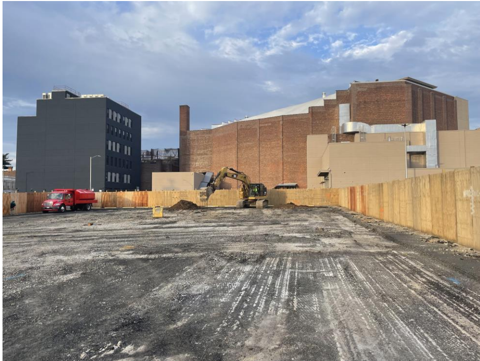
Photo 1: View of excavation for SOE installation along the perimeter of Lot 14, facing east.
