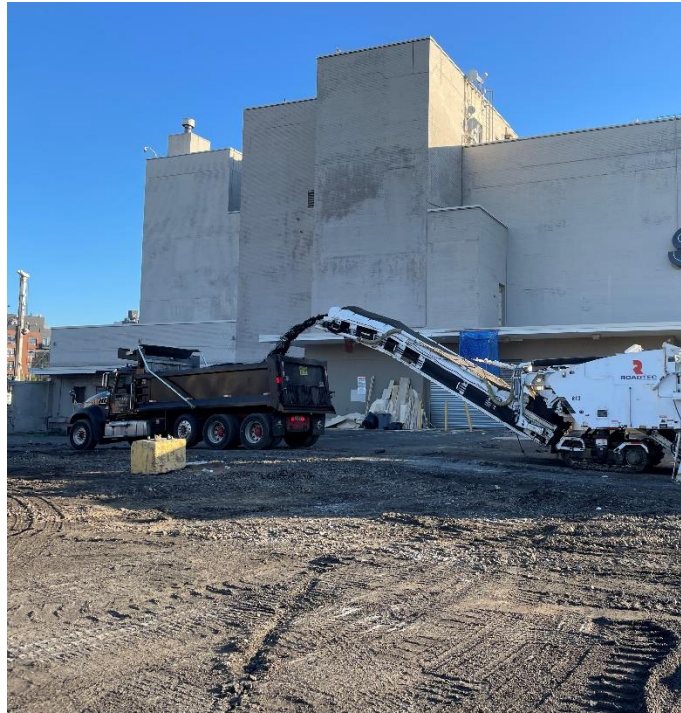
Photo 1: View of asphalt stripping in Lot 14, facing south.
