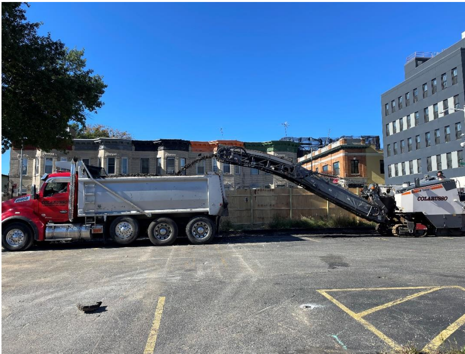
Photo 2: View of asphalt stripping, facing west.
