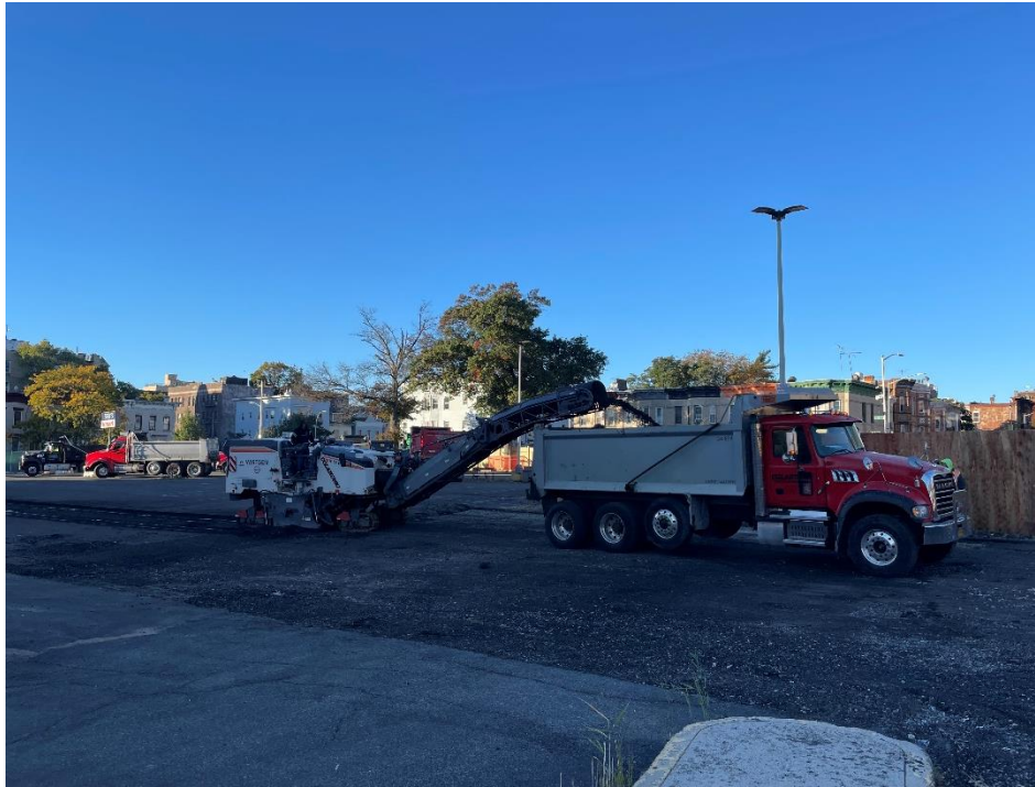
Photo 1: View of asphalt stripping in lot 14, facing southwest.
