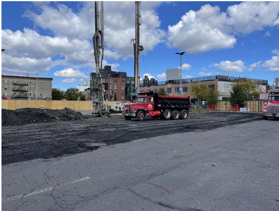
Photo 2: View of asphalt stripping on Lot 14, facing northeast.
