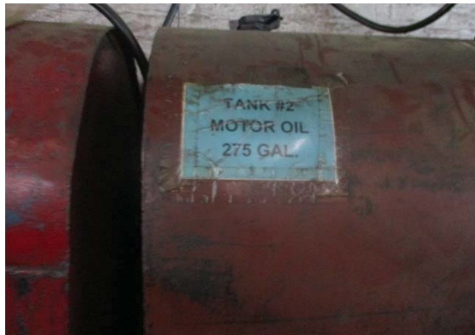
Above-ground storage tanks
