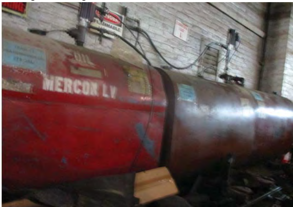
Above-ground storage tanks
