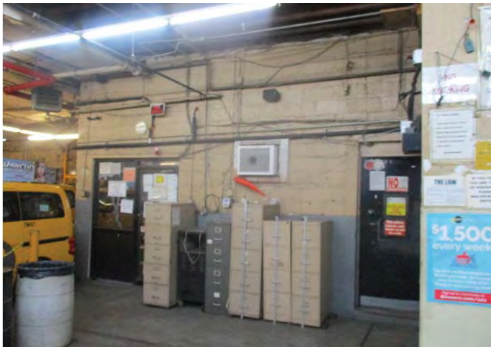
Wall mounted A/C unit
