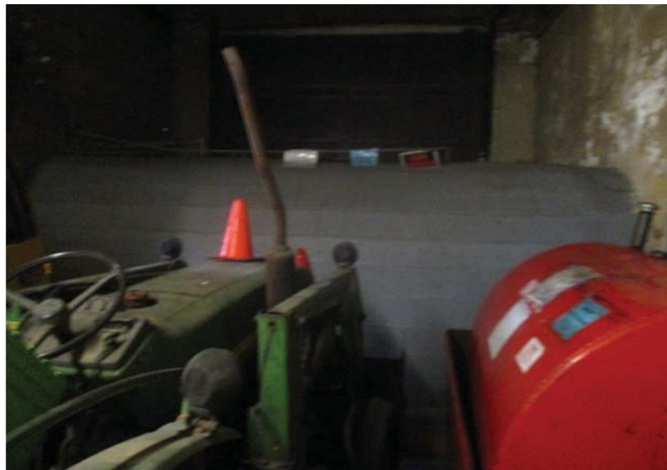
Fuel oil and waste oil UST's
