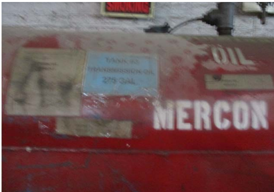
Above-ground storage tanks
