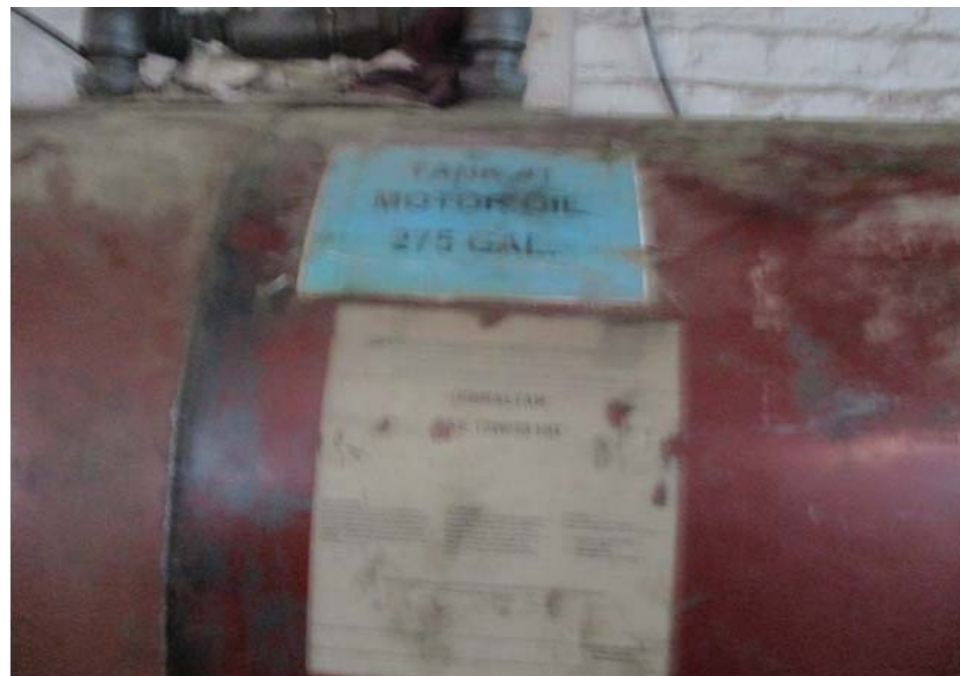
Above-ground storage tanks
