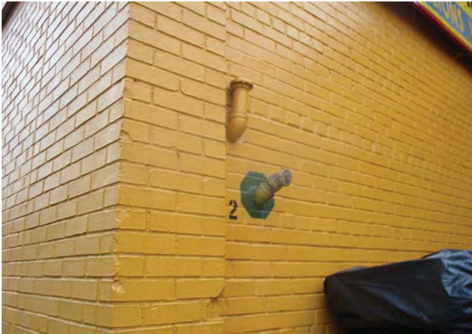
Fuel oil tank fill and vent
