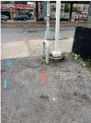
Picture 5: ELECTRICAL AND WATER COMING FROM THE STREET.
