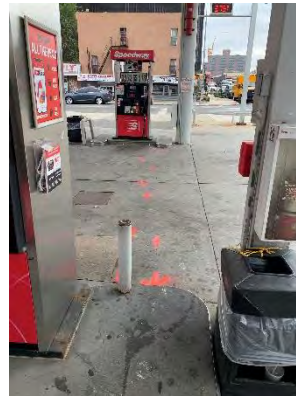
Picture 6: ELECTRICAL GOING TO THE PUMPS.
