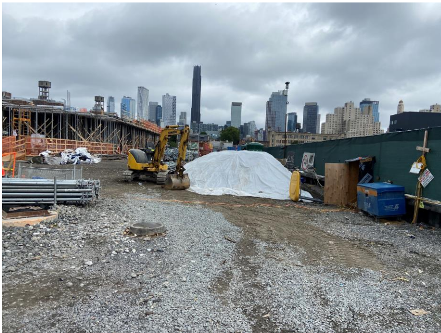
Photo 2: View of stockpile covered with polyethylene sheeting within the SPW (facing north)
