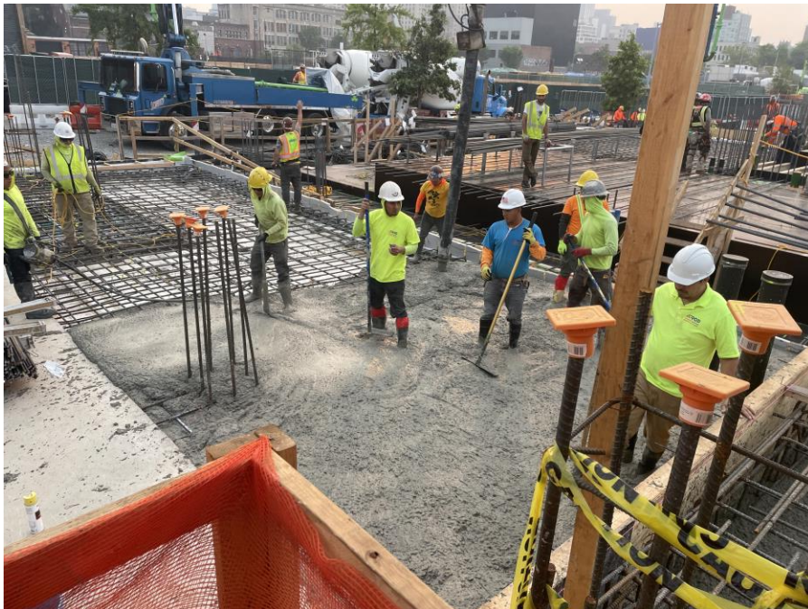
Photo 2: Kingdom placing concrete for the first-floor slab in the northeastern part of Society Brooklyn (facing northeast)
