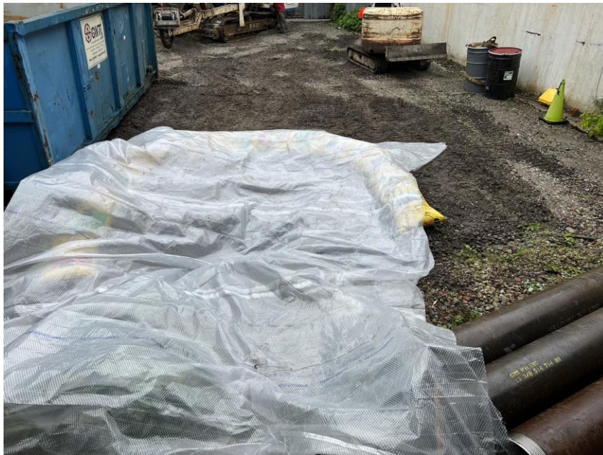
Photo 2: Polyethylene sheeting-lined sump at P-2 and settling tank in the northern part of the site (facing northwest)
