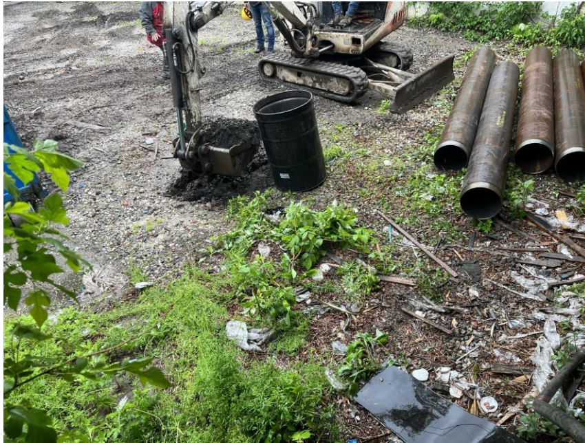
Photo 1: Allstate 12 excavating a temporary sump and placing soil/fill into drums in the northern part of the site (facing west)
