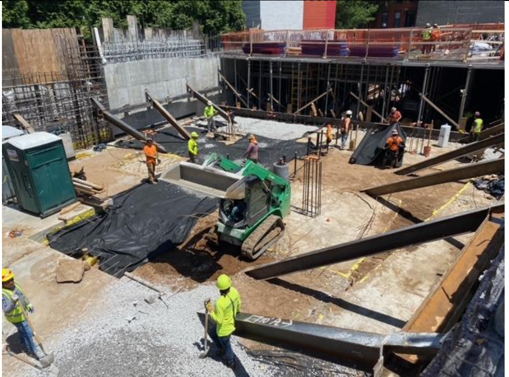
Photo 4 – Facing Northeast Grading of stone and placing initial layer of geotextile layer..
