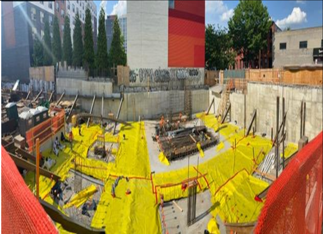
Photo 3 – Facing North Laydown of chemical vapor barrier on eastern portion of the Site.
