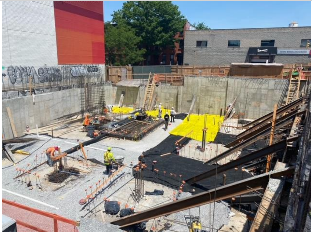
Photo 2 – Facing Northeast Compacting, grading and installing 2 nd geotextile layer above chemical barrier.
