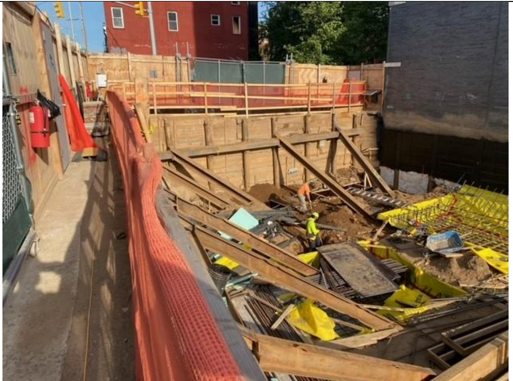
Photo 2 – Facing Southeast Digging along the West wall for the footer tie in (CAMP 1 Station shown in the corner)
